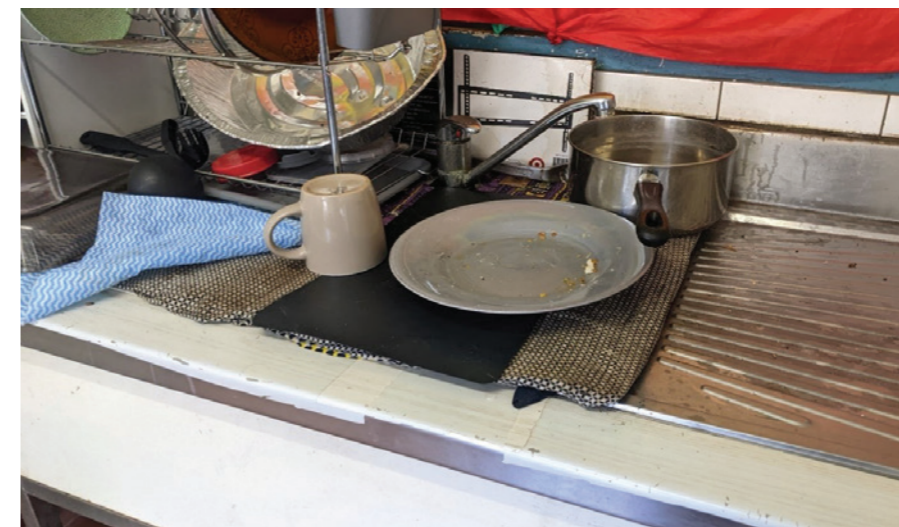
↑ Broken sink and householder work-around. Image. Liam Grealy
