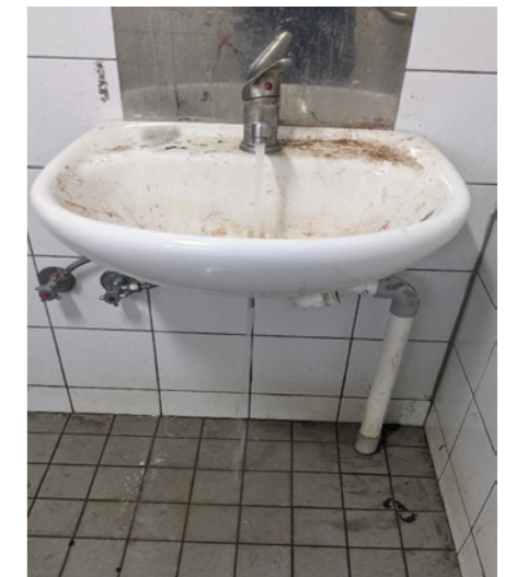
↑ Sink water flows onto the bathroom floor. Image. Liam Grealy
